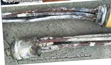
Pipe joint fittings had to be replaced because of scale and rust.
