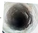
2 weeks after Vulcan was installed, scale had been softer and fallen out.
