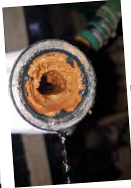
First inspection: May 21, 2018. Inside of a secondary small pipe, before Vulcan S25 was installed.
