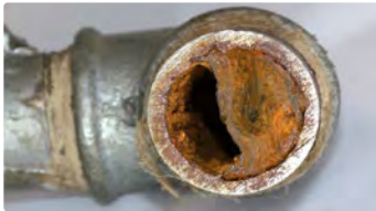
Pipe with limescale deposits
