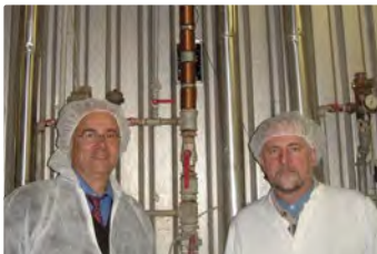
Vulcan installed in a food factory
