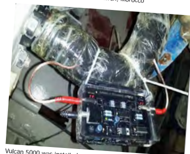
Vulcan 5000 was installed on the water inlet of the water recycling room.
