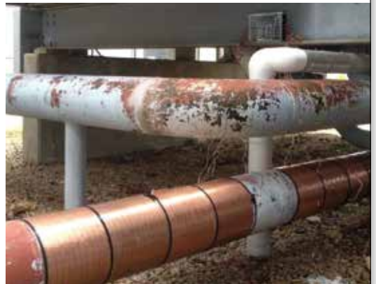
Vulcan S250 installed on a 10 inch diameter line that feeds twin cooling towers (CT-1 and CT-2)
