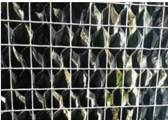
The photo above was taken of CT-1 about 3 weeks after the Vulcan was installed.
