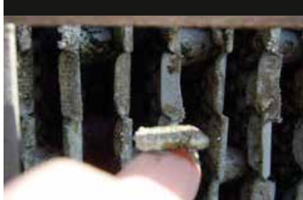
Silica could not be removed by the high pressure water gun, but can be peeled off with a nail.
