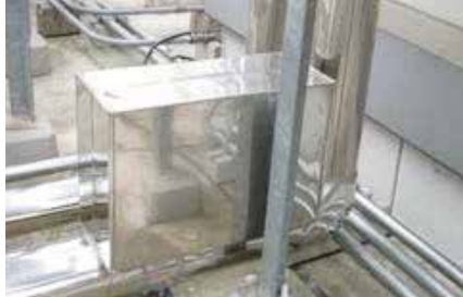
Vulcan S25 was installed on the makeup water pipe for the cooling towers A, B and C.
