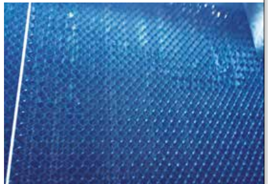
The inside of CT-1, after 3 weeks with Vulcan. It illustrates clean flutes that are in constant contact with Vulcan-treated water and a few dry (untreated) areas that still have some remaining green biofilm.
