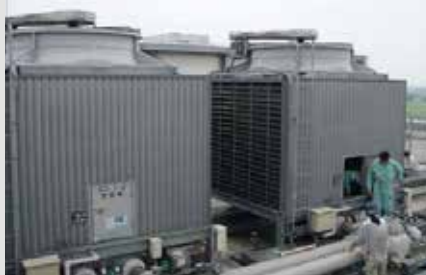
Cooling Tower A Cooling Tower B
