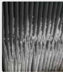
Cooling tower grids
