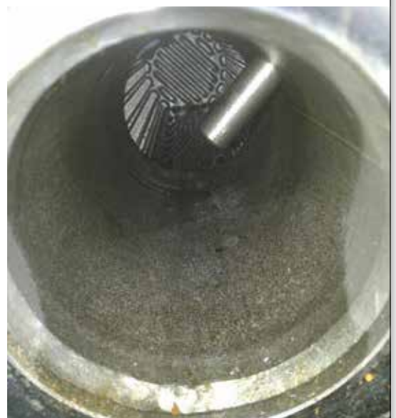
After 3 months – with Vulcan treatment. Up to now the installed pipeline needed no cleaning.
