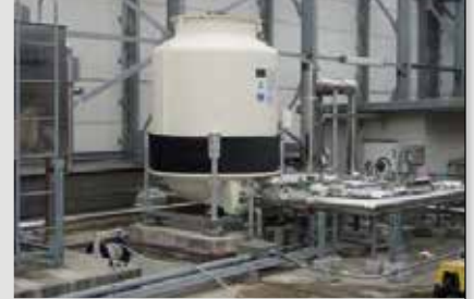
Cooling Tower C
