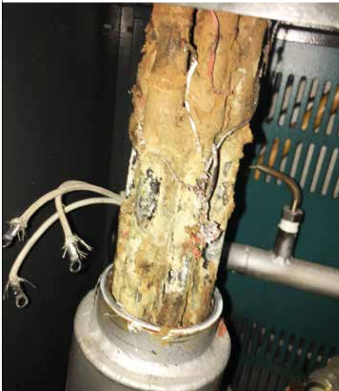
Untreated heat exchanger for 3 years.
