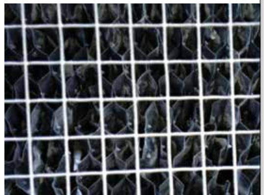
The photo above was taken of CT-1 about 6 weeks after the Vulcan was installed.
