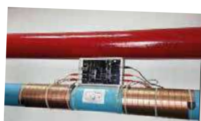
Anti-Scale System Vulcan S25 installed
