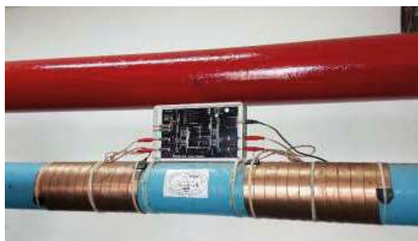
Anti-Kalk System Vulcan S25 installiert
