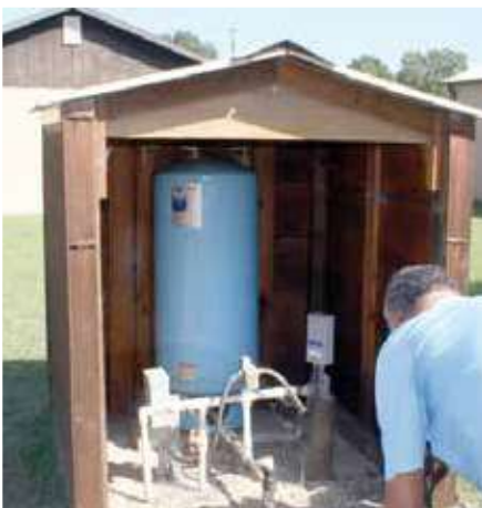
Home well water system
