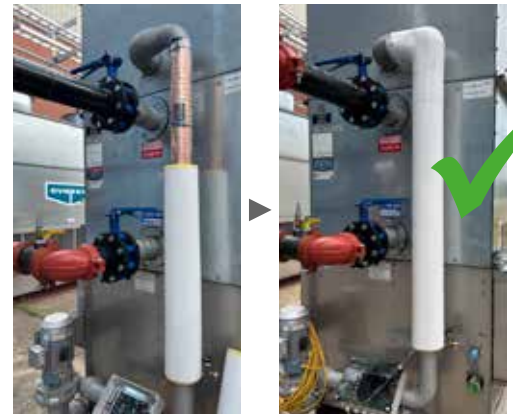
Outdoor pipe insulation to protect the impulse bands.
