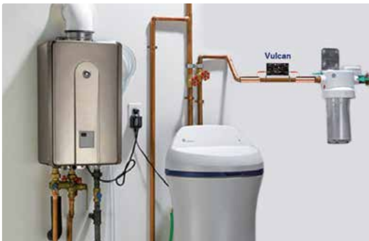
Vulcan installation with a water softener
