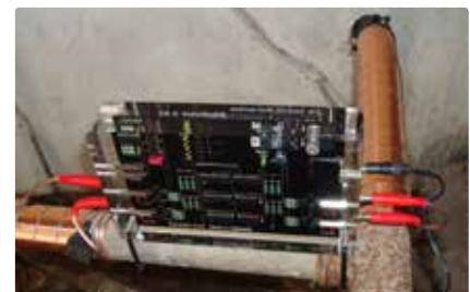
Vulcan installation in an apartment building
