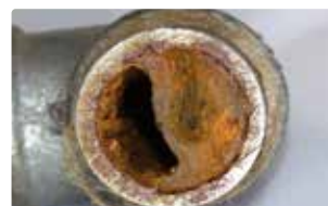
Pipe with scale deposits
