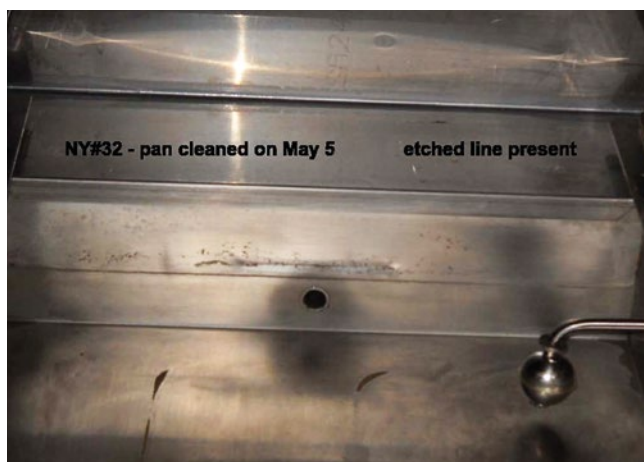
After Vulcan installation — pan area is now completely scale-free. There is a slight indentation into the pan at the waterline.
