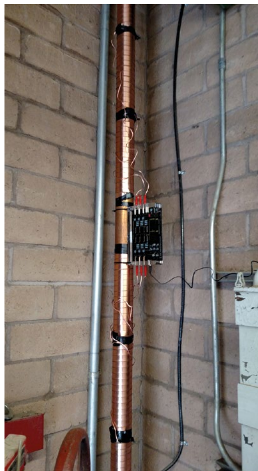
Vulcan S100 installed on the main water line
