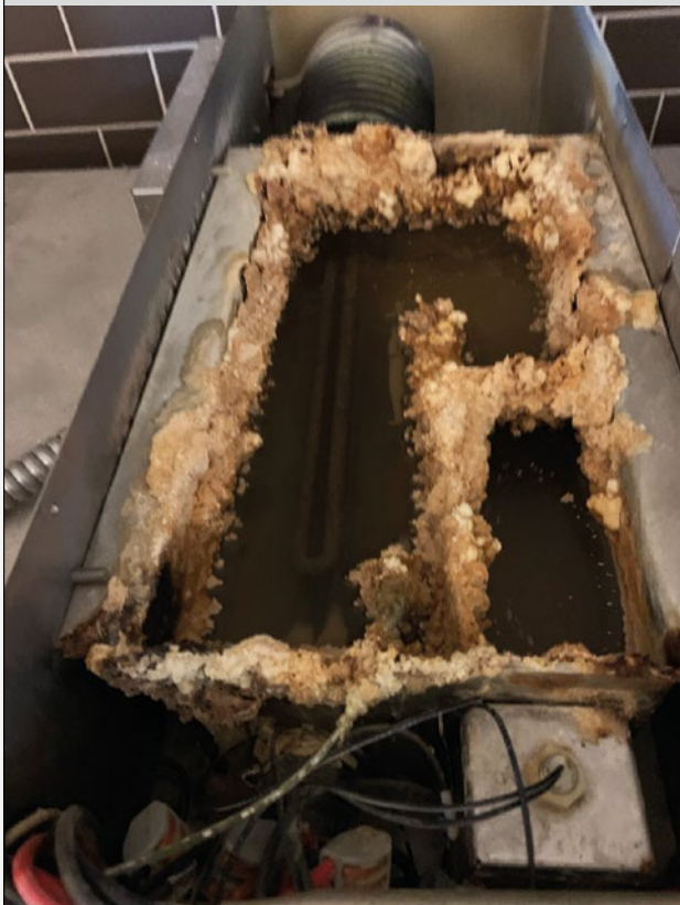
The bread oven before Vulcan installation. The scale deposits were cleaned and Vulcan 5000 was installed.
