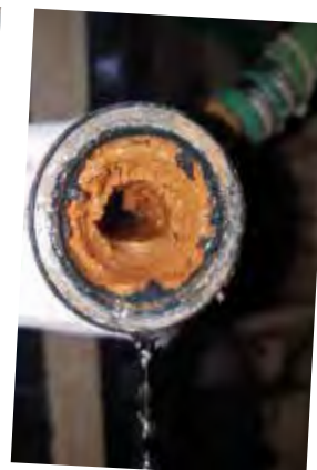
First inspection: May 21, 2018. Inside of a secondary small pipe, before Vulcan S25 was installed.
