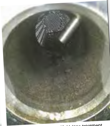
After 3 months – with Vulcan treatment. Up to now the installed pipeline needed no cleaning
