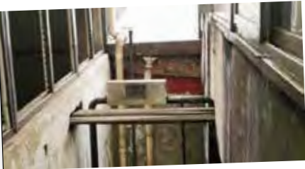
Vulcan S25 outdoor installation
