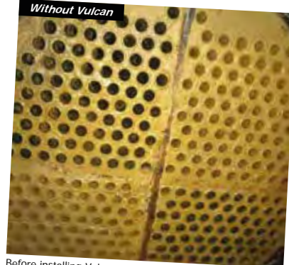
Before installing Vulcan, the scale was very thick and hard in the heat exchanger tubes.
