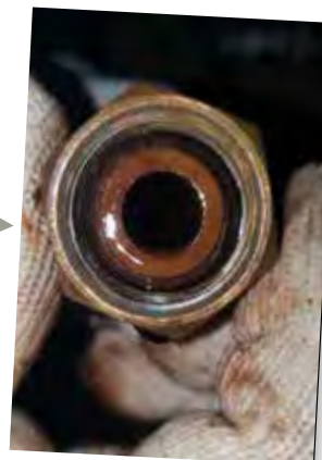
Last inspection: November 21, 2018. After 6 months with Vulcan treatment: the pipe is free of scale.
