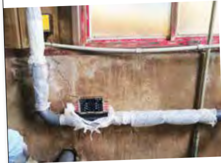
Vulcan S100 was installed in the sewage room to treat the sludge dewatering machine.
