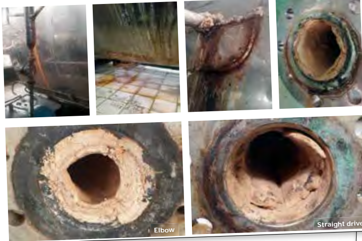
Hot water return pipe to the exchanger for cooling
