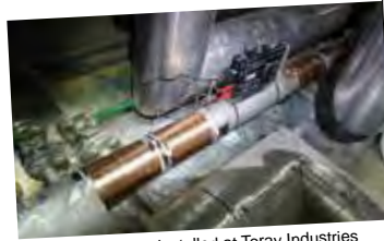
Vulcan S25 installed at Toray Industries
