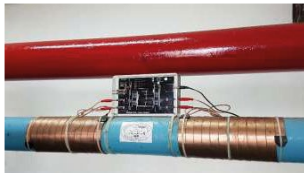
Anti-Kalk System Vulcan S25 installiert
