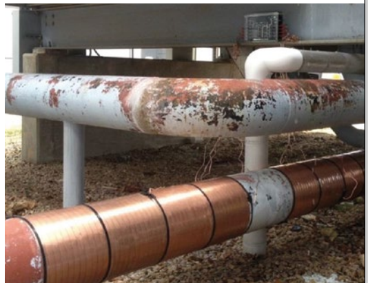
Vulcan S250 installed on a 10 inch diameter line that feeds twin cooling towers (CT-1 and CT-2)
