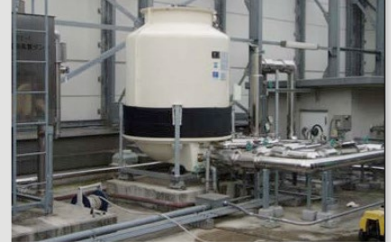
Cooling Tower C
