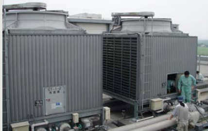
Cooling Tower A Cooling Tower B
