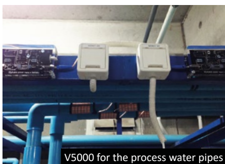
V5000 for the process water pipes
