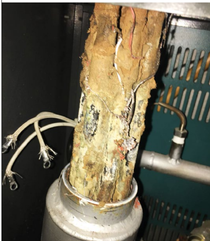
Untreated heat exchanger for 3 years.
