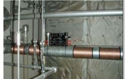
Vulcan S25 was installed on the circulating water pipe for the cooling towers C.
