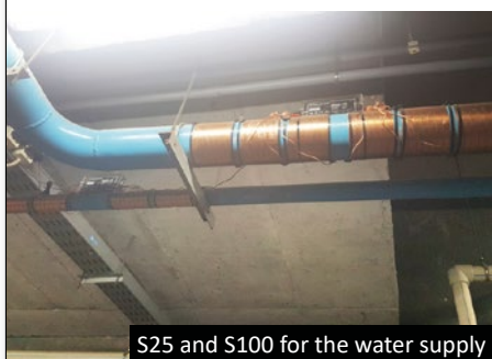
S25 and S100 for the water supply
