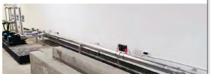
1 set of S100 installed for the air-source heat pump water heater in apartment building 10
