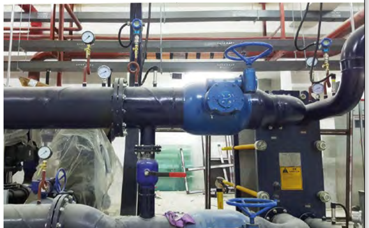
Vulcan S150 was installed in the heating system in the low zone of the heat exchange station.
