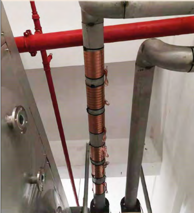
1 set of S100 installed for the air-source heat pump water heater in apartment building 1
