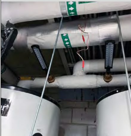
Vulcan S10 was installed on the hot water recirculation on the 27th floor. The impulse bands were covered to prevent condensation before the Vulcan unit was installed.
