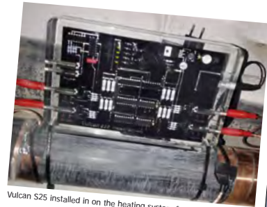
Vulcan S25 installed in on the heating system for 132 apartments
