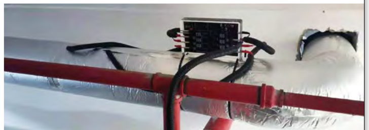
1 set of S100 installed for the air-source heat pump water heater in apartment building 2
