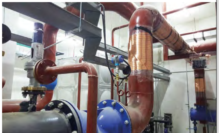
Vulcan S350 was installed in the heating system in the high zone of the heat exchange station.
