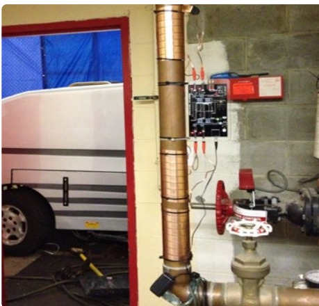
Vulcan S25 Installation in der Ice Land Eishockey Halle
