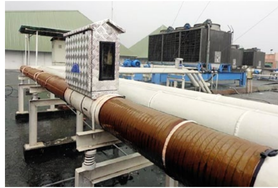
Vulcan S500 was located inside aluminum box and installed on a cooling tower main pipe.
